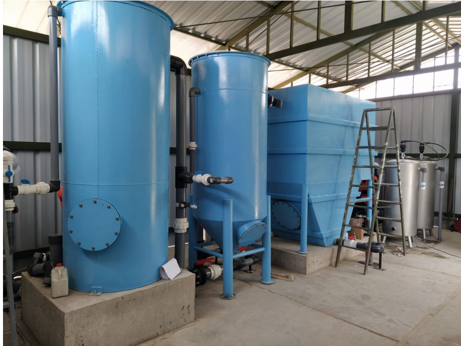
Plant in operation Community of Tala – Torata – Moquegua Q_{max} = 0.70 - 2.0 lt/sec AngloAmerican Quellaveco
