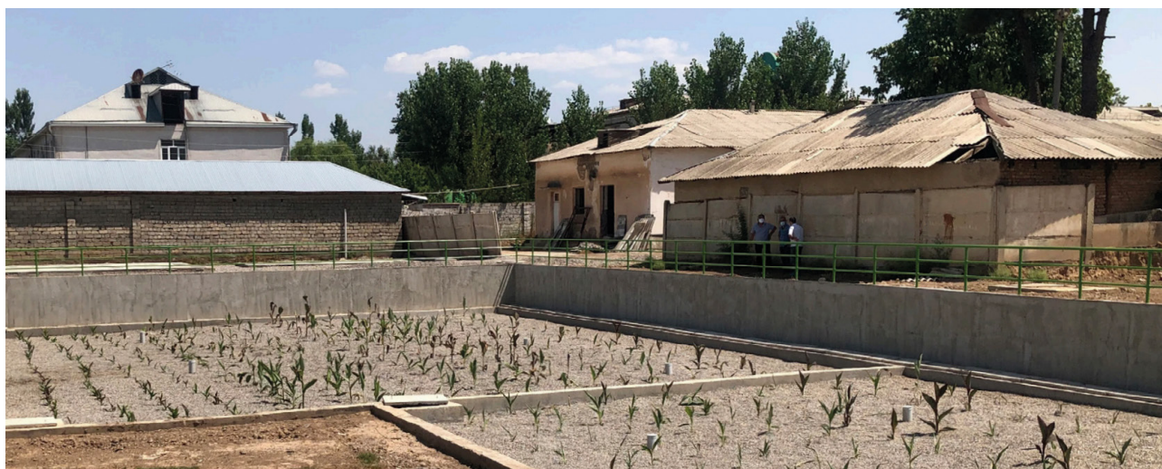
► Figure 3. DEWATS has three main treatment steps and modules: primary treatment, secondary treatment, and advanced secondary treatment options. The figure shows a completed DEWATS with planted gravel filter, an advanced secondary treatment option ( Ali, 2022 ).
