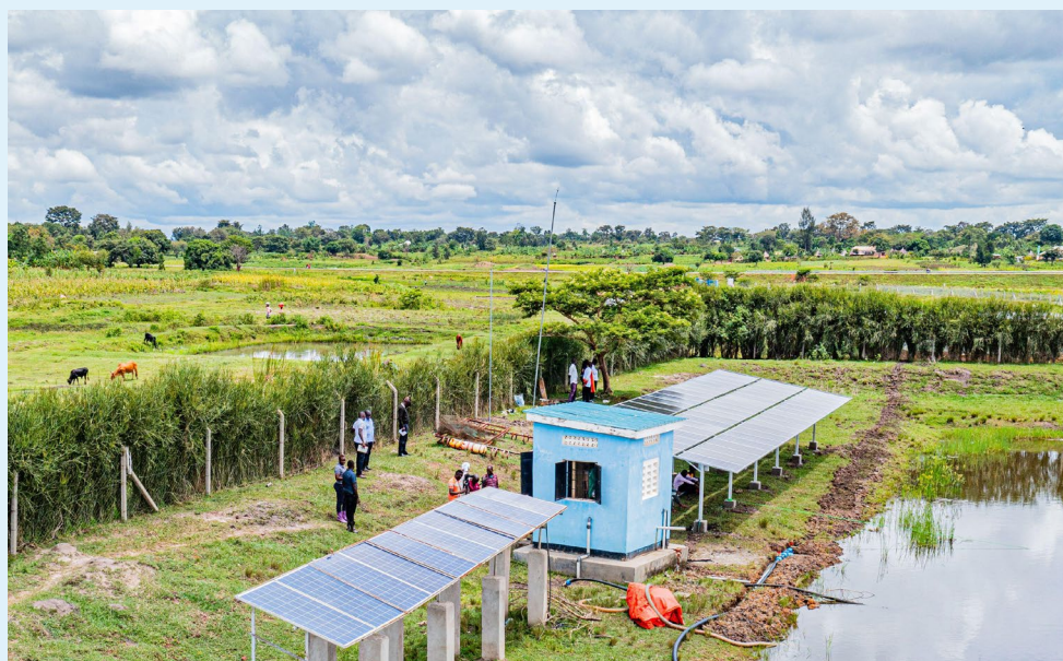
► Figure 8. A solar-powered pumping station providing irrigation water for agriculture in Kumi District, Eastern Uganda © Amazing Aerial / Alamy Stock Photo
